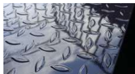
Tear plate on the floor
